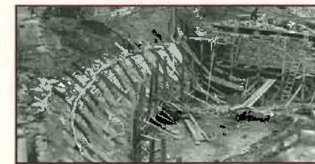
Circa 1942 photograph of Churchville Reservoir Dam under construction. Source: Courtesy of the Churchville Nature Center .
